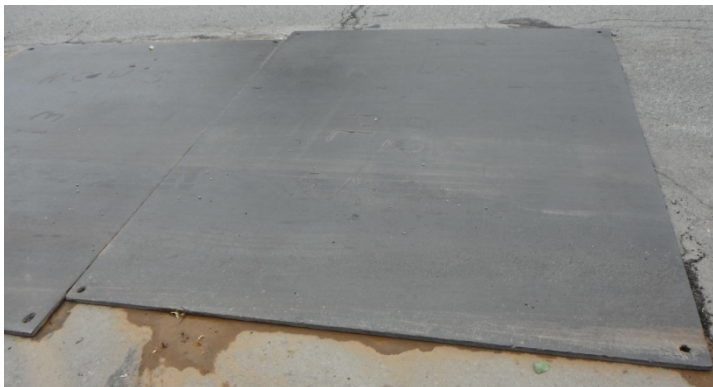
Exhibit 2: Unpinned and Unramped Street Plate.
