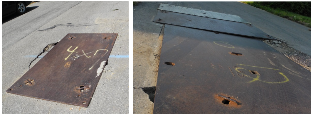
Exhibit 3: Excavations Not Fully Covered by Street Plate.
